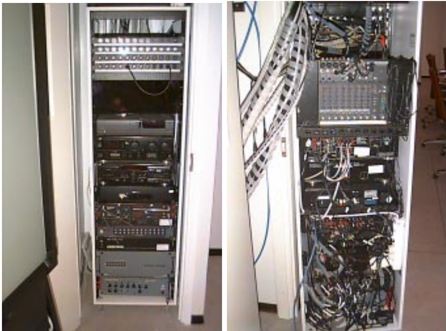
Figure 3. The heart of the Studio – the front and back of the equipment tower.
